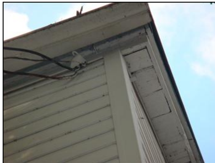
2. cable covered with siding
