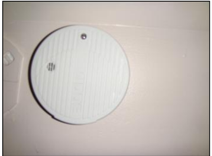
5. not working 2nd floor
