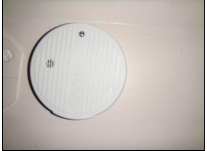
16. not working 2nd floor
