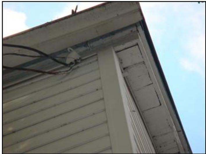
12. cable covered with siding
